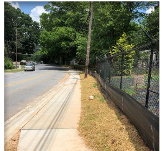
SPLOST-funded improvements made to the sidewalks at North Druid Hill Road and Valley Brook Road. Work is underway to transform the corridor into a multimodal-friendly complete street supporting various uses.
